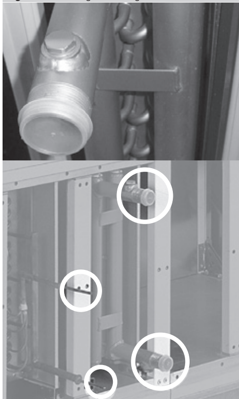
Figure 16 – Heating and cooling media feed
